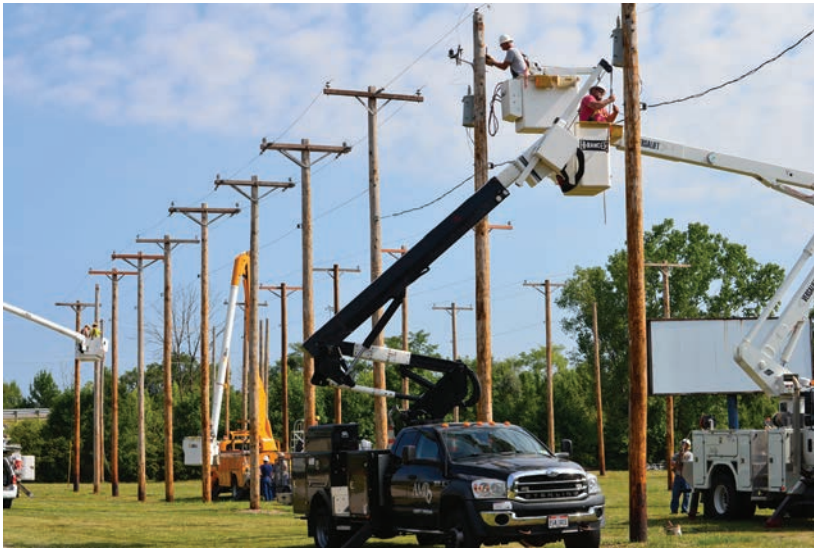
Volunteers help prepare the de-energized pole field for the upcoming Lineworkers Rodeo.
